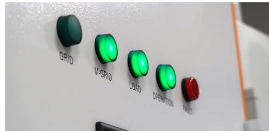
Microgrid control system
