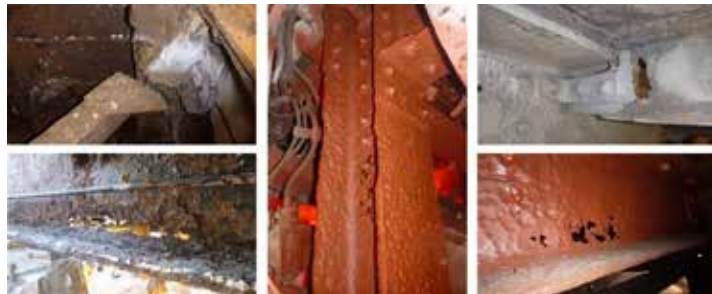
What was found under when investigated... holing, severe section loss, heavy pitting and failures.
